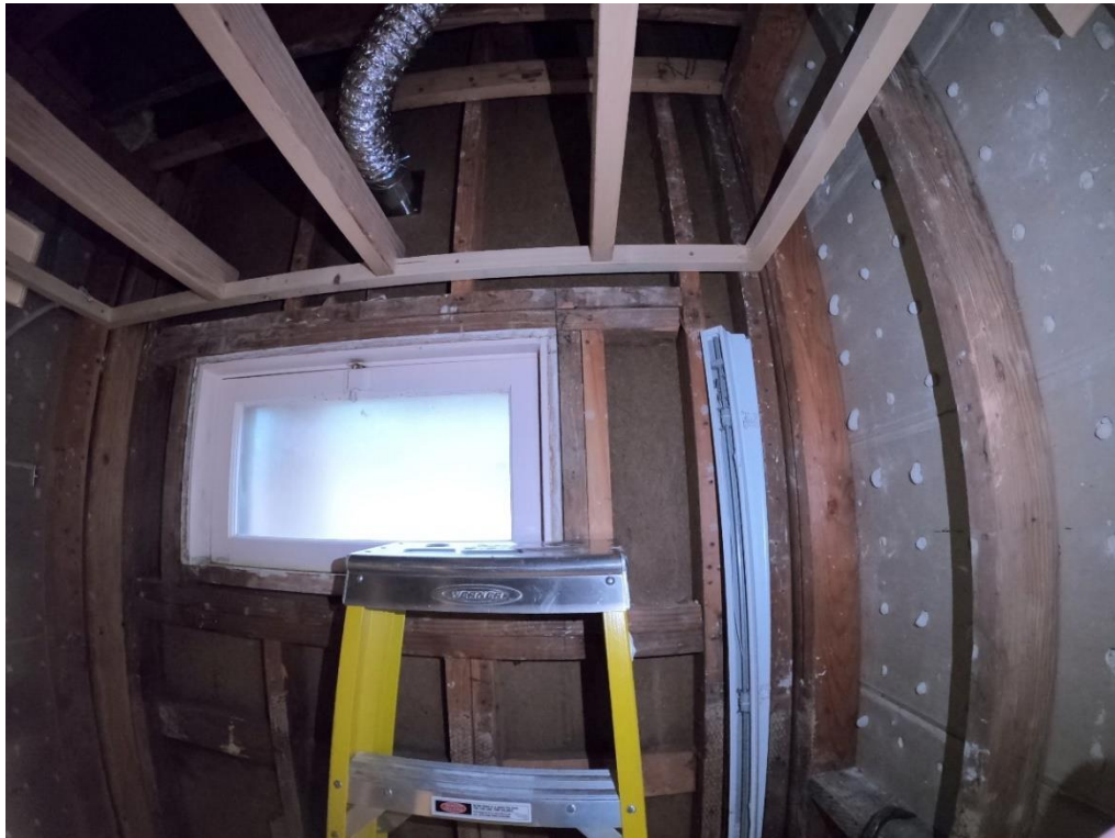
Original Hospital Exterior Wall with missing header and wood fiber wall sheathing at West wall
