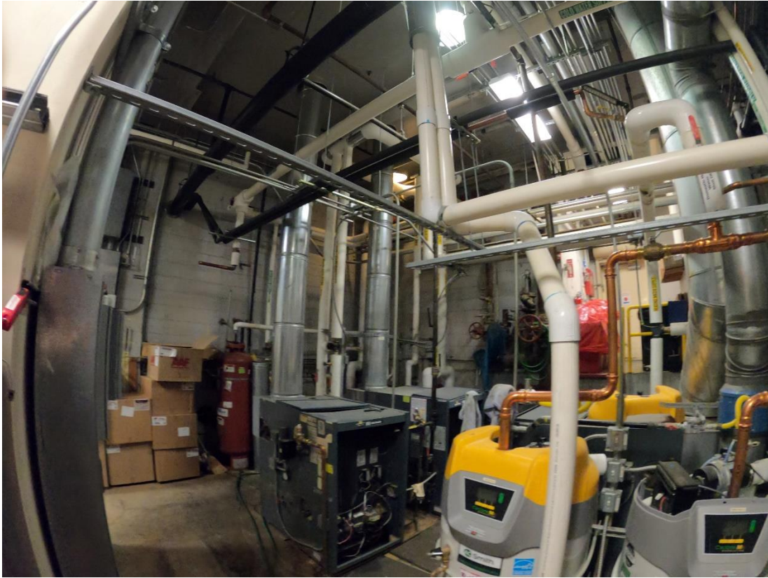
Original Hospital Boiler Room with unbraced piping
